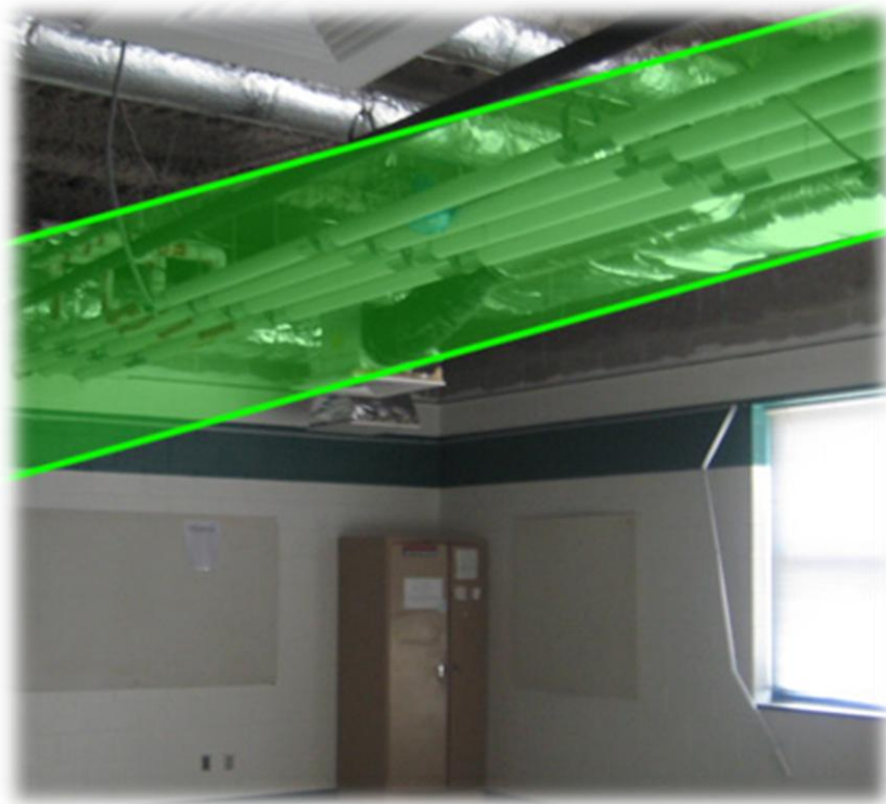
Figure 7: Installed Pipe Insulation
