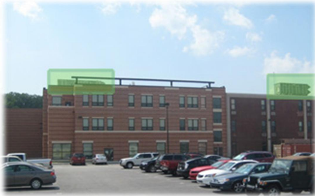
Figure 5: Rooftop AHU without screens
